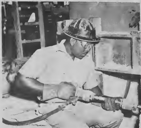
GOGGLES meant the difference between an injured eye and a normal employee. While breaking concrete last month a chip flew into his eye goggles took the impact. He wasn't even scratched.
